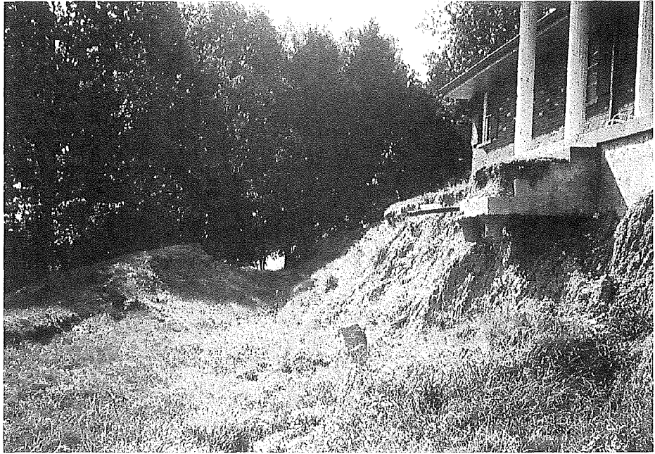
This type of damage can result when improper grading or site preparation occurs.
